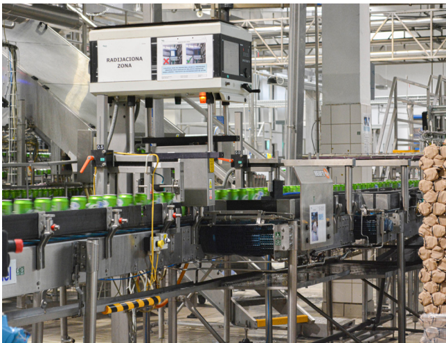
Sustainable work process in can filling line.
