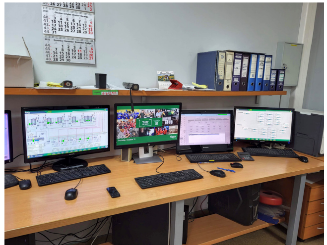
Energy management and cooling systems.
