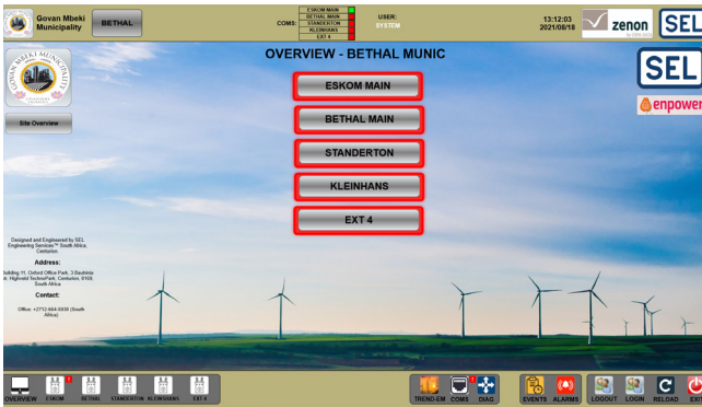
Operators can now see all networks in the Bethal Municipality, including recent events, alarms and trends.
